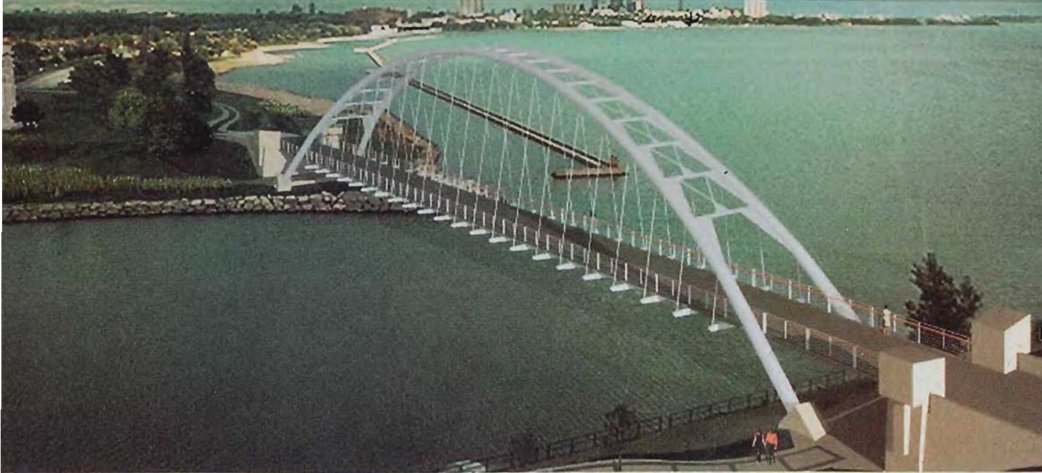
SOFT SOILS dictated need for enormous caissons for bicycle-pedestrian bridge. Image by Richard Szegidewicz.
